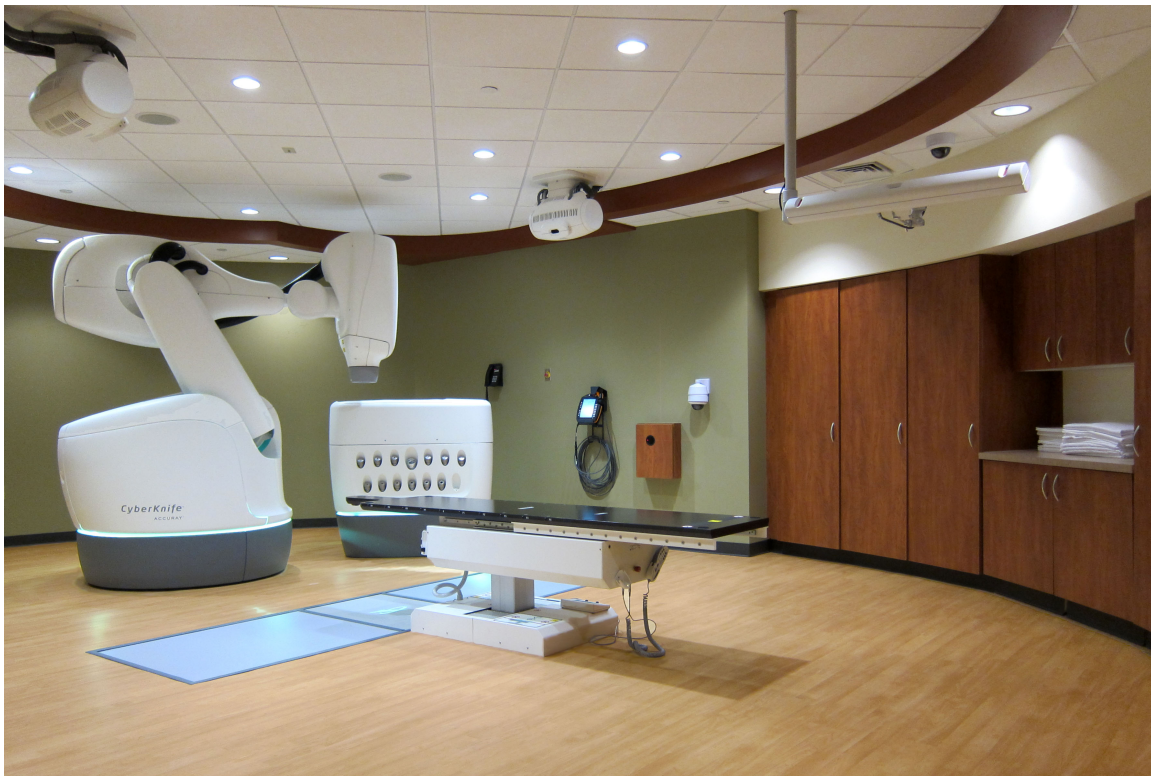
Figure 4.2.1 Typical treatment room setup for CyberKnife M6 Installation
